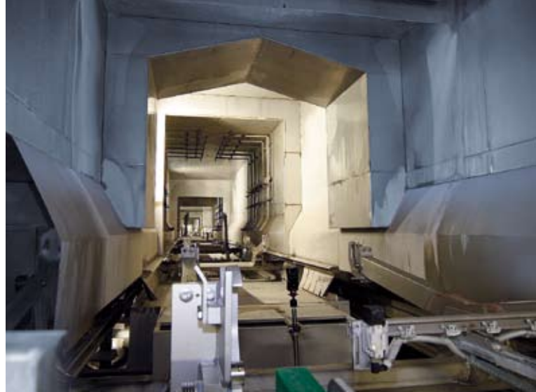
Pretreatment inlet gateway
