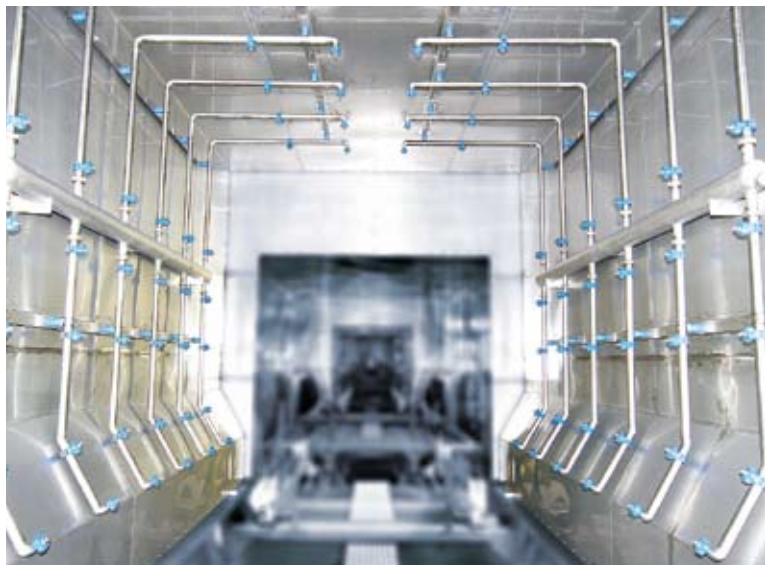
Rinsing area with spray rings
